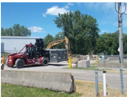
Workers begin the process of loading soil that was excavated when installing the site's permeable treatment wall.
